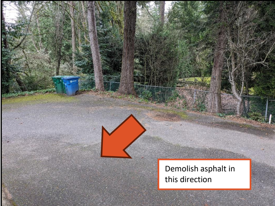
Photo 4. Base of tree 38 viewed from the south. The driveway is proposed for removal in this area. I recommend the asphalt removal begins closest to the tree and moves backwards. Once the pavement is removed no machinery traffic or materials are allowed. I recommend the project arborist is called if any large roots over 2-inches diameter are encountered.
